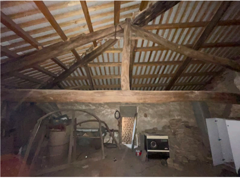
d Detail of the attic room truss, you can notice the irregularity and cracks of the wood
